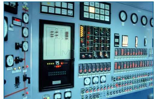
McNeil Generating station control room Courtesy of DOE/NREL
